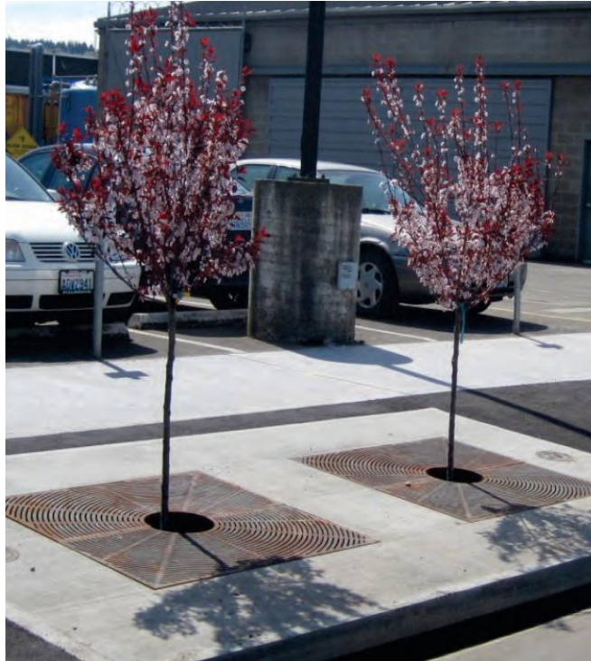
Figure 5 - Filterra® Bioretention System installed adjacent to sidewalk
