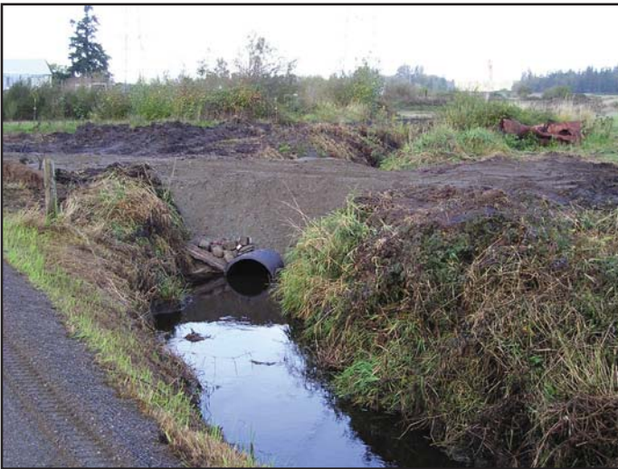
Undersized culvert with unstable road crossing
