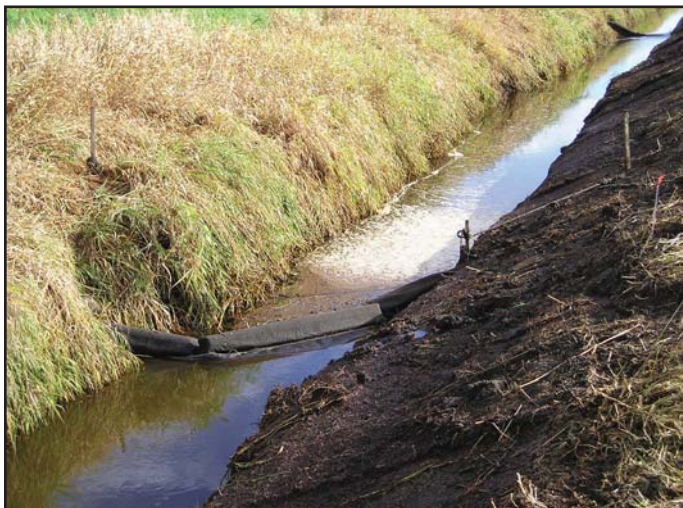
Temporary silt fence
