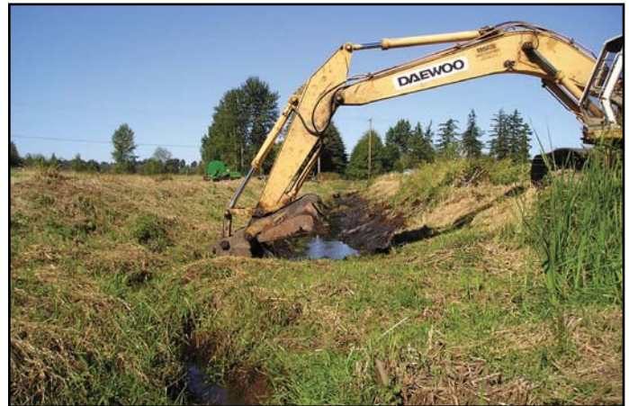
Drainage Maintenance can be a significant source of sediment release
