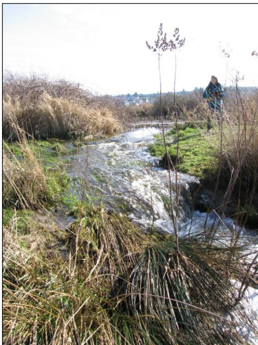
Figure 15 – New Jones Creek channel crossing old farm road (13 March 2006). Jo Gardiner is standing on the old farm road immediately SE of plot 12, following the failure of the Jones creek culvert.
