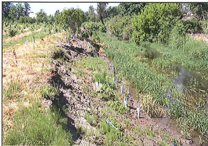
Bank Failure following herbicide application
