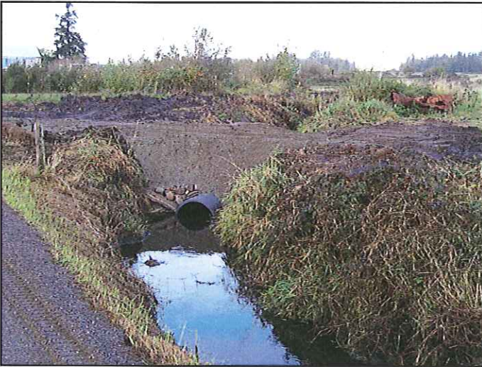
Undersized culvert with unstable road crossing
