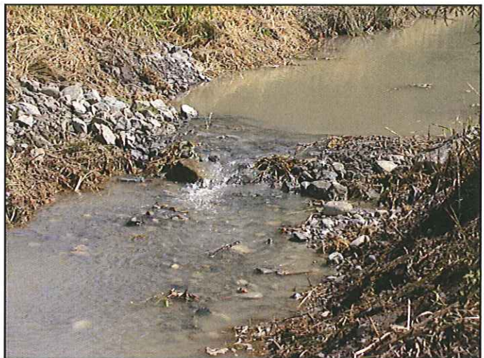
Simple Coffer Dam slows the water flow allowing sediments to settle
