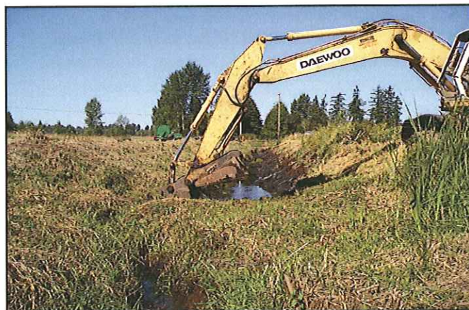
Drainage Maintenance can be a significant source of sediment release
