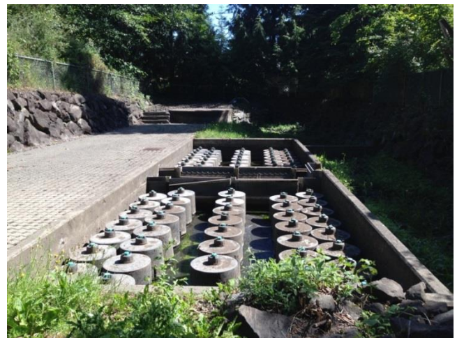
Giles Ave Treatment Facility (May 2017)
